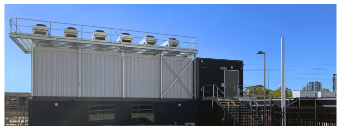
eCentre micro data centre for NEXTDC in Australia
